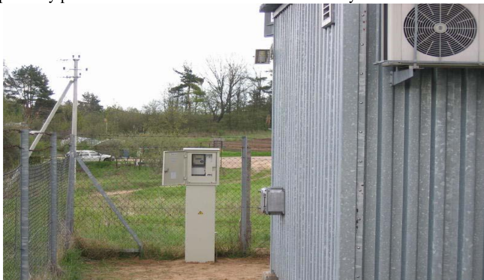
The positioning of a power metering pillar on the territory of the receiving-transmitting system of a mobile communication system operator
