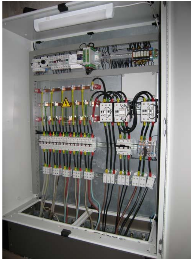
Fig. 1. A street lighting power supply unit
